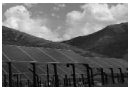
Above: Solar panels cover the shade structures on the new facility's pens. Photo: The Marine Mammal Center
